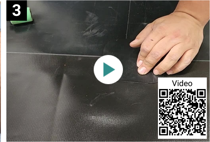
3 Follow video to show how to get nozzle into position and how to use roller while welding.
